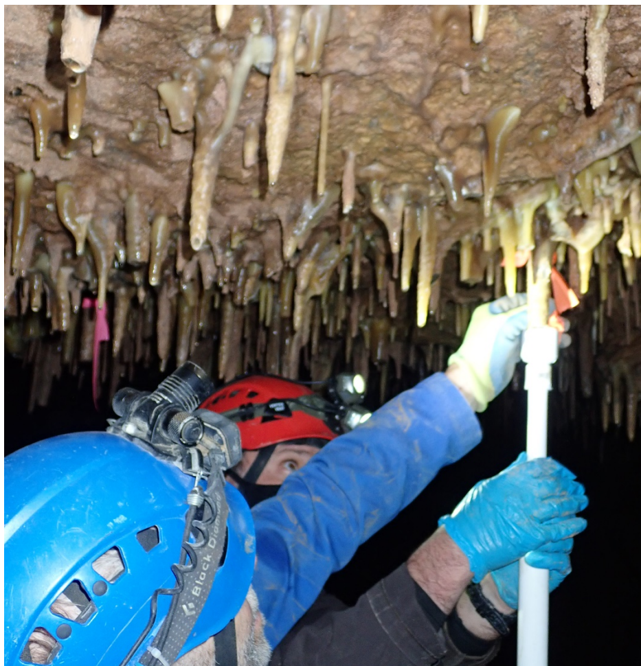
Mike and Knutt positioning a Stalactijack under a repair. Note in the upper left the broken formations we have not found matches to.
